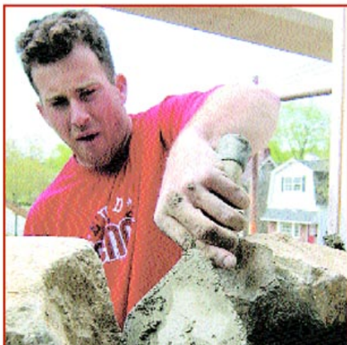
PITCHING IN. Steve Bonitatis of DCN Construction replaces stonework on the south wall of the Black Horse Inn in Hometown. A variety of local employees and businesses have been doing improvement work at the inn lately, including Ferguson Painting Contractors, which recently painted the building with materials donated by Sherwin Williams. Springfield Township staff pitched in to power-wash the inn from top to bottom a few weeks ago. DCN Construction is repairing the south wall that was inadvertently damaged last summer, working around a couple of new window frames that were custom built free-of-charge by local preservationist Dick Meyer.
